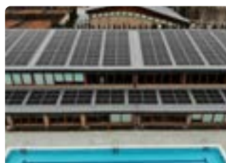
David Lloyd – solar PV installations
