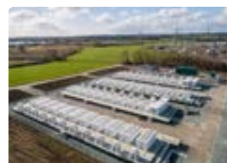
Pillswood – battery storage
